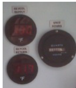
14: Temperature Gauges & Hour Meter
