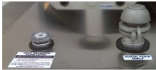
32: HTF Level Gauge & Vented Filler Cap
