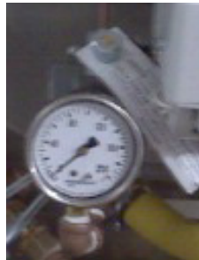
26: Fuel Oil Pressure Gauge (PSI)
