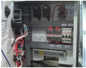
9: Control Panel, Inner
