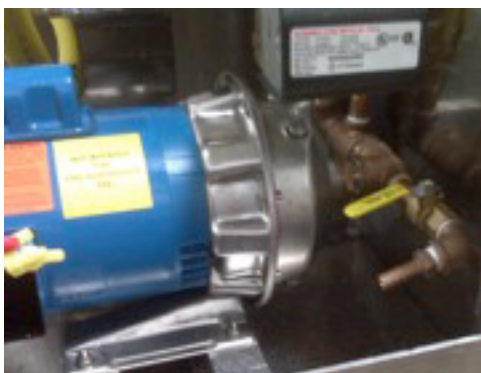
6: Fluid circulation Pump
