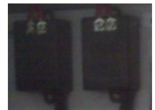
18: Transformers for Digital Temp. Gauges
