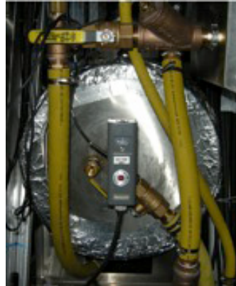
33: HTF Circuit Valves, Y-strainer & High Temp. Limit
