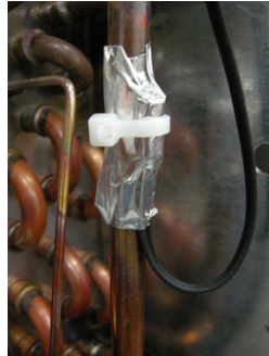
Thermistor attached to the refrigerant line.
